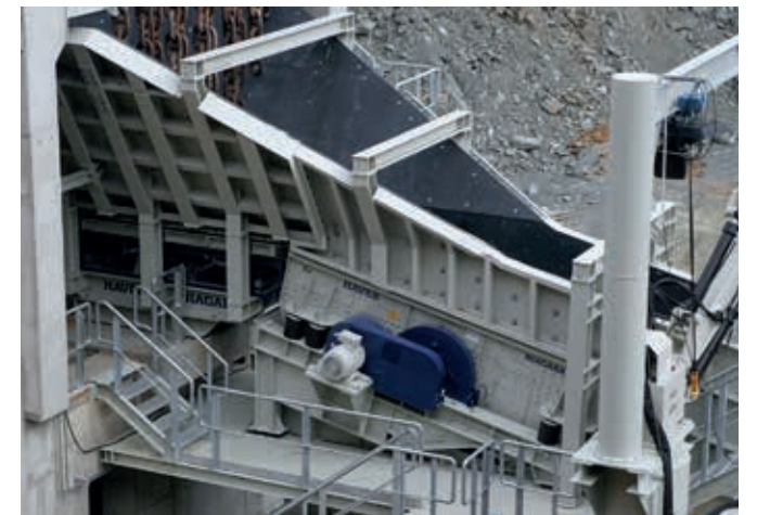
Rugged bunker construction using the HAVER reciprocating feeder
