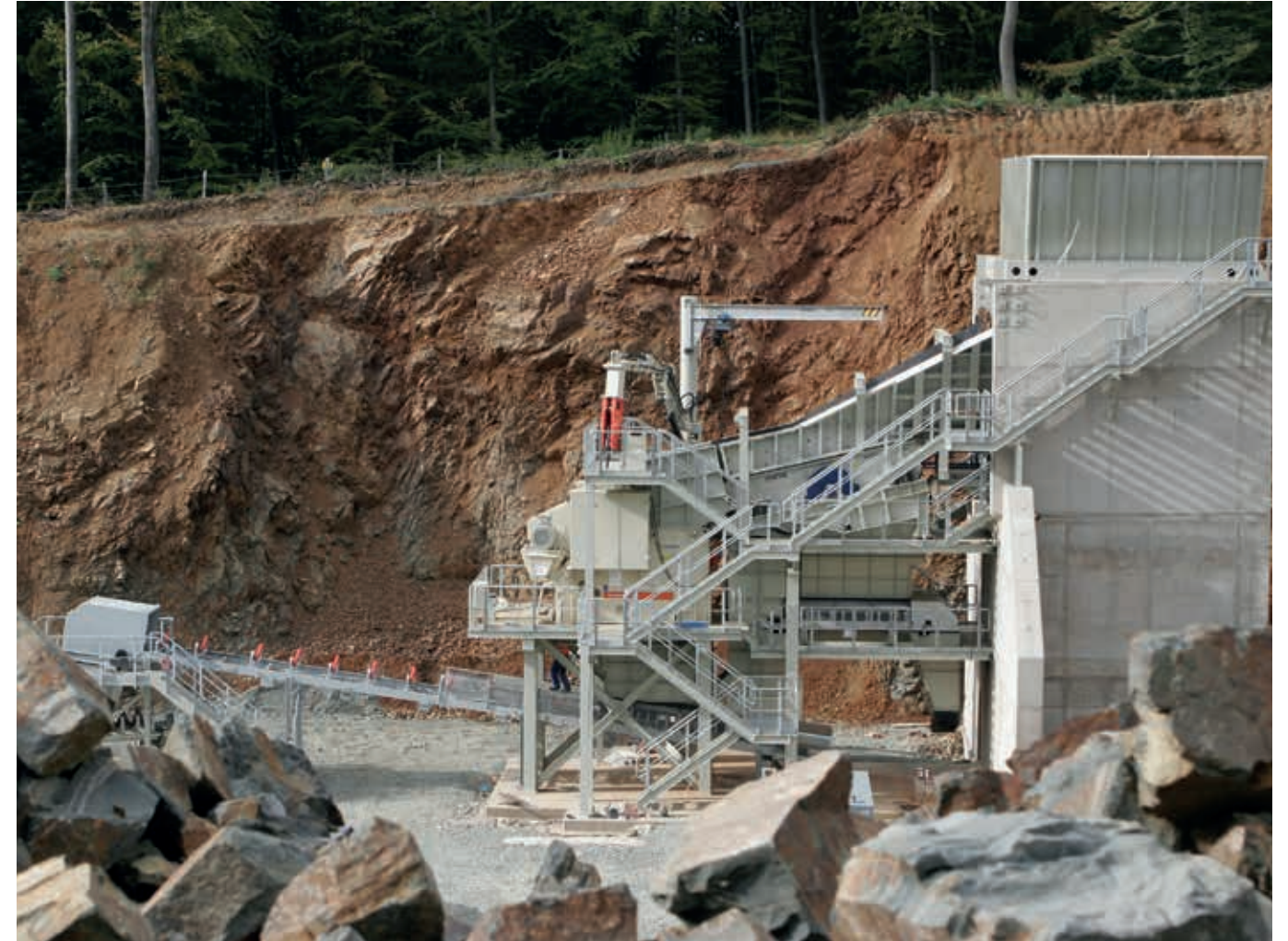
BASIC Primary crushing plant, diabase, 500t/h, HAVER F-CLASS, HAVER push feeder, jaw crusher
