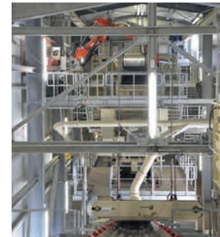
Primary crushing plant, raw gypsum, 400t/h, HAVER F-CLASS, apron conveyor, jaw crusher
