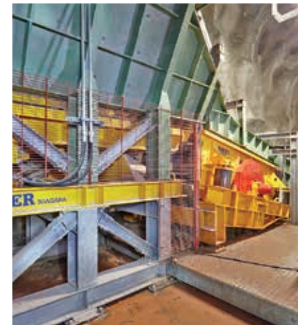
Primary crushing plant, flourspar and feldspar, 80t/h, HAVER F-CLASS, HAVER push feeder, jaw crusher
